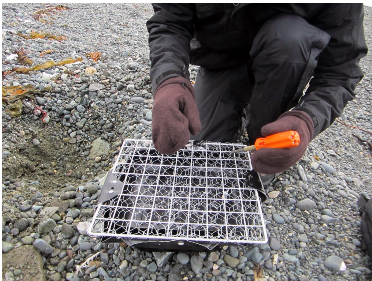
Figure 11: Opening the top mesh of the PED ROCK to shovel rocks into the center. Note the hole is already dug in this photo.
